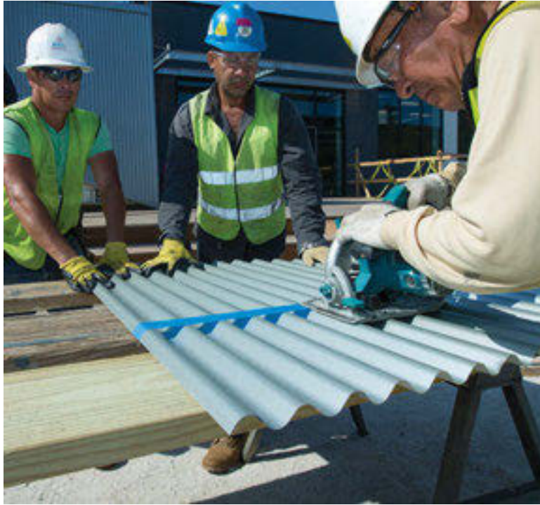
Workers from Capstone Contracting Co., a subcontractor on the Open Works' project, cutting corrugated metal panels.
