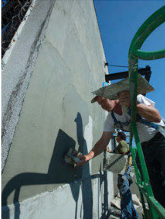
The Coastal Exterior Services Inc. crew applies stucco to repair the facility's east-facing façade.
